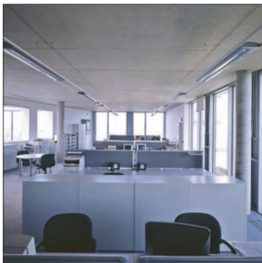
Exposed slab in Offaly County Council building. Architect: ABK Architects. Source: Christian Richters
