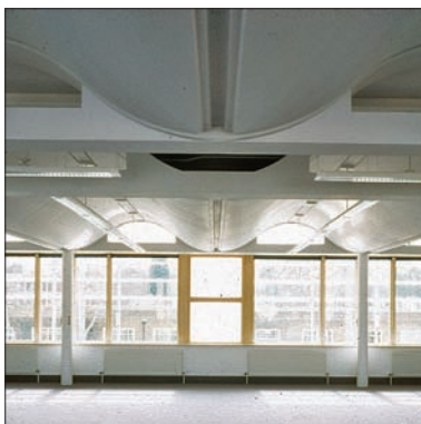
Sinusoidal slab in the BRE building, Watford. Architect and source: Fielden Clegg Bradley Studios
