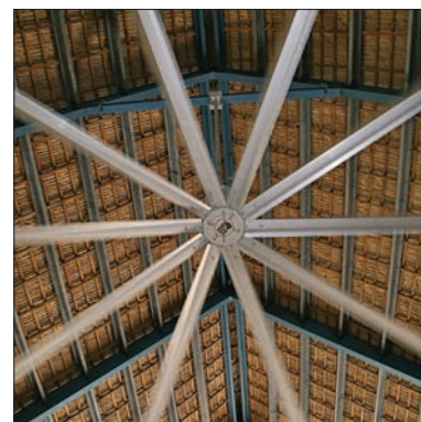
Ceiling fan providing air movement. Source: Passiefhuis Platform VZW (PHP)
