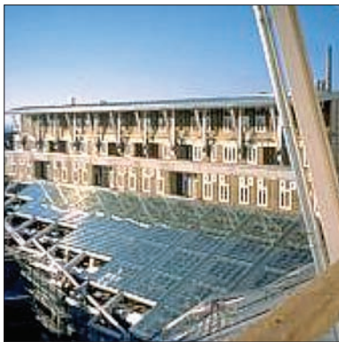
Integrated photovoltaic roof in Prisma, Nurnberg. Architect and source: Joachim Eble-Architektur
